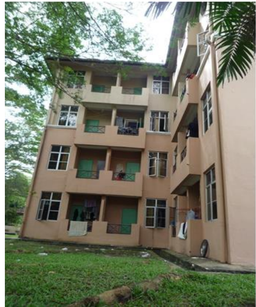
(c) Casement and turn window design with tinted glass and large balcony in each residential unit faces to outside areas
